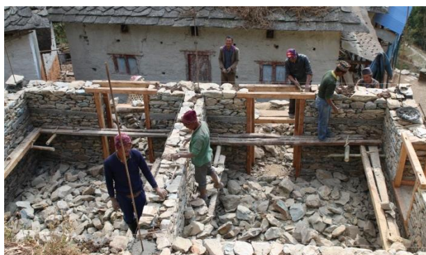
Community members work together on an earthquake-resilient house at Bijulikot, Ramechhap. © Medair/Wendy van Amerongen
