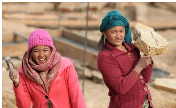
Two masons work on the reconstruction of earthquake-resilient houses at Bijulikot, Ramechhap. © Medair/Wendy van Amerongen
