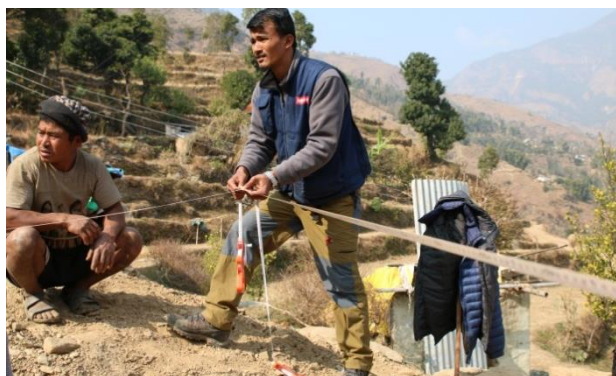
Medair and masons work on the layout of an earthquake-resilient house at Bijulikot, Ramechhap. © Medair/Wendy van Amerongen
